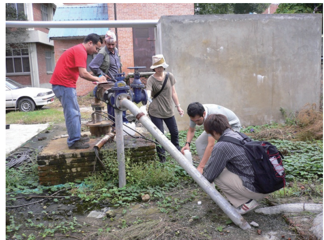
At a deep well in a city area.
